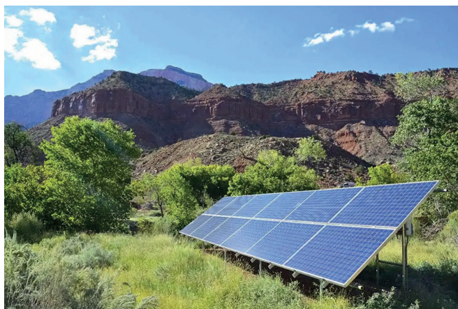
Figure 7. Solar panels installed on the ground [5]
