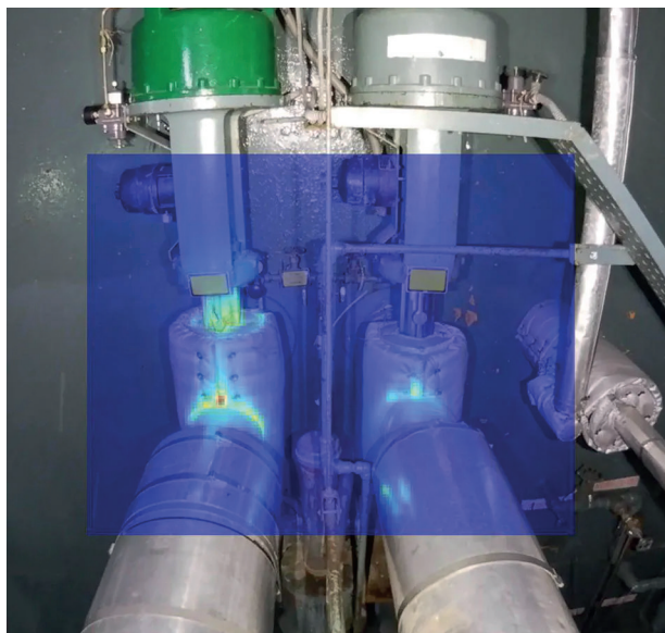
Figure 6. Thermal camera image showing a pipeline leak [11]
